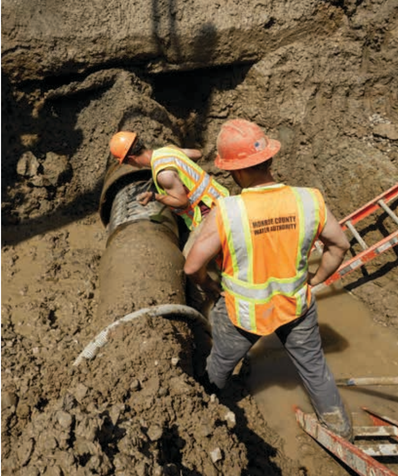
To appreciate the vastness of our system, consider we maintain 3,477 miles of water mains, 27,514 hydrants, 50 water storage facilities (48 tanks, 2 reservoirs), and 48 pump stations.
